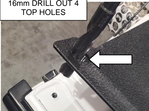
ENLARGE HOLES TO 21mm
